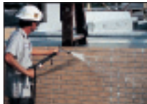
Panel is cleaned to remove concrete leakage.
