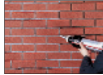
Mortar is installed into the brick joints with a grout bag or with mortar dispensing gun.
