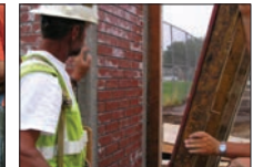
Forms are removed and the finished wall is power-washed to reveal a classic brick or stone finish in the structural concrete wall.
