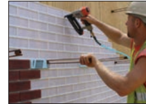
Rim snaps tab together and are stapled on a vertical surface to create a template to hold brick.
